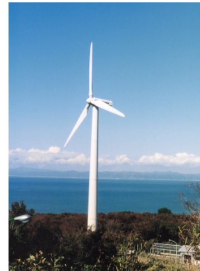
An installed example of wind power generation equipment (400 kW) under the interest subsidization program
