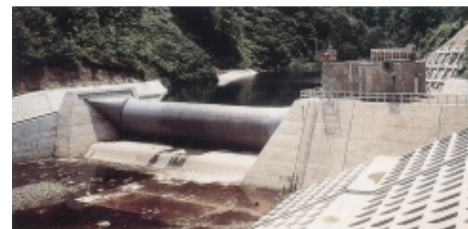
Relief weir made of rubber-coated fabric at the Kurotani Power Plant
